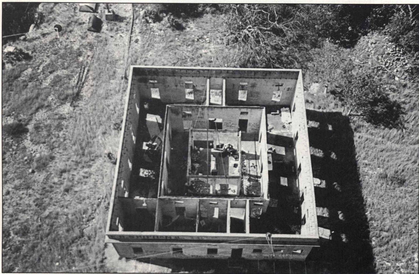
Dating back to the turn of the century, the old Navassa Light keepers quarters is in a sorry state of disrepair.
